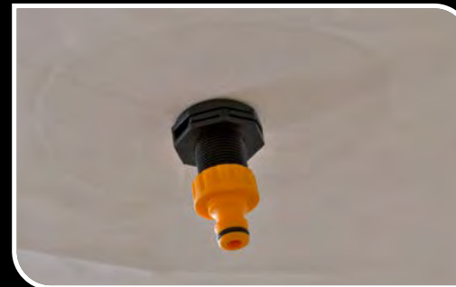
Central Drainage Point
